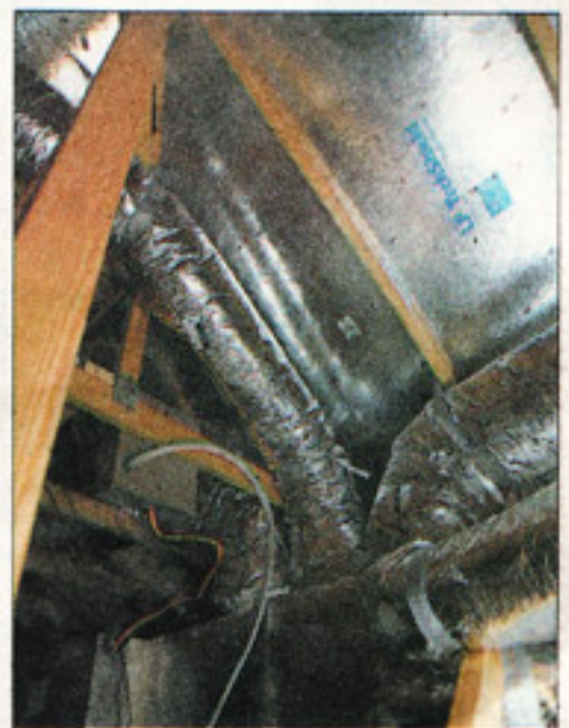
Armadillo Homes uses radiant barrier roof decking and well-insulated ductwork in the Energy Star-rated homes its building in Stonecreek.
